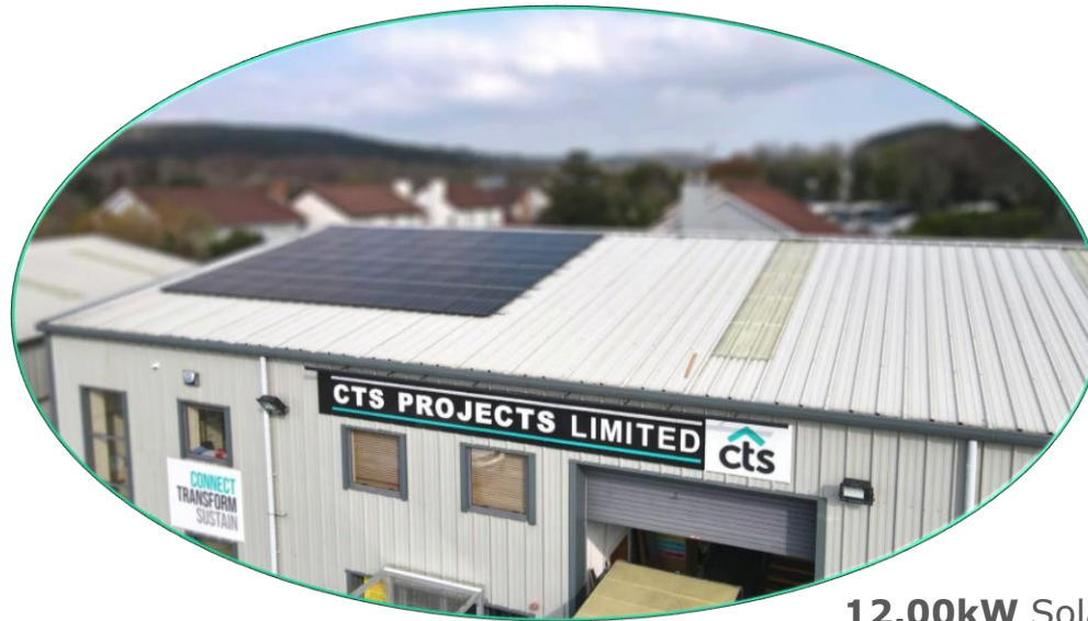
12.00kW Solar PV Array (CTS, Warrenpoint)
